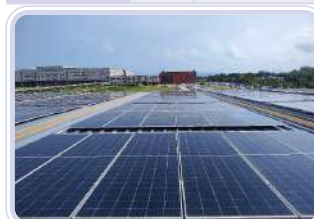
Rooftop solar energy
