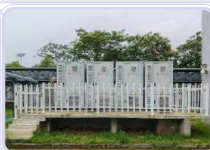
Energy storage cabinet
